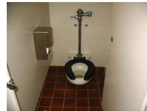
Toilet Fixture in Food Services Building
