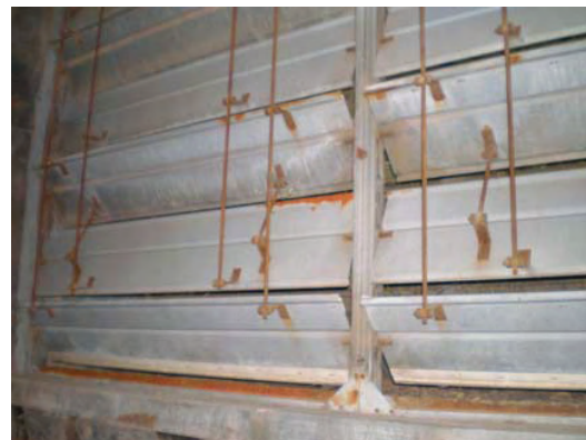
Natatorium Vent'l System – OA Dampers
