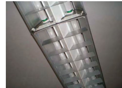
Existing Lighting in Humanities
