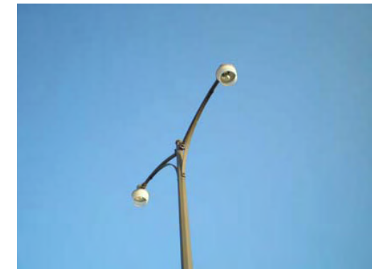
Parking Lot "Cobra Head" Fixture
